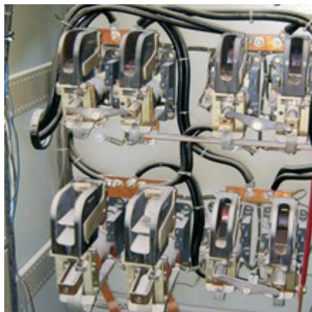
Traditional DC contactors
